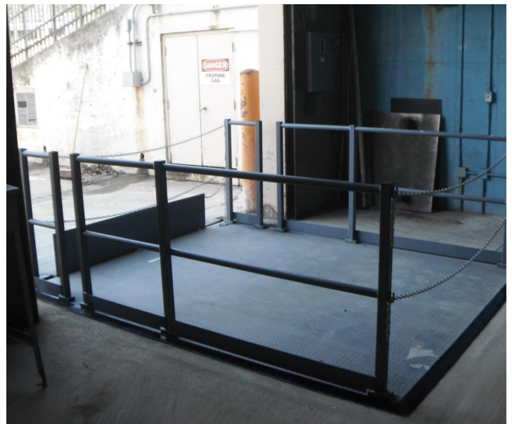
New dock lift in closed position with railings and access chain
