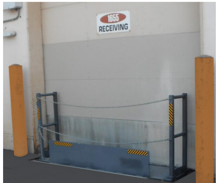
Exterior view - overhead door closed and new dock lift lowered - showing safety rail door cut out
